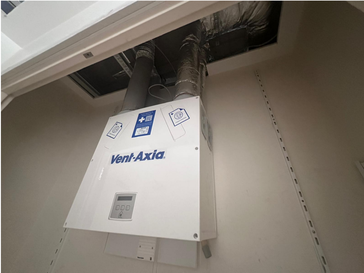
New MVHR Units Installed
